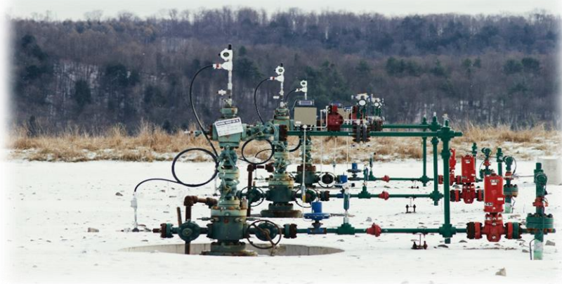
Natural gas well heads on well pad
