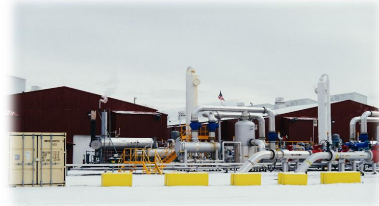
Edsell compression station in Chaffee Corners
