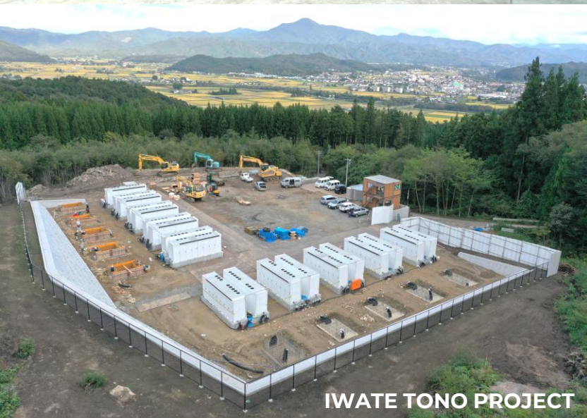
DP NEXT PRODUCTION PLANT
