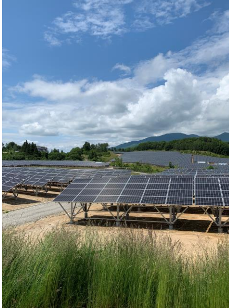
The 26-MW Nari Aizu Solar Power Plant in Fukushima
